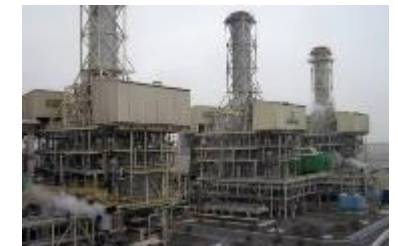
Waste Heat Recovery
