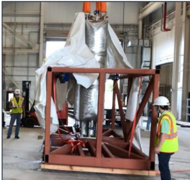
Low Temperature Recuperator Heatric, Inc.
