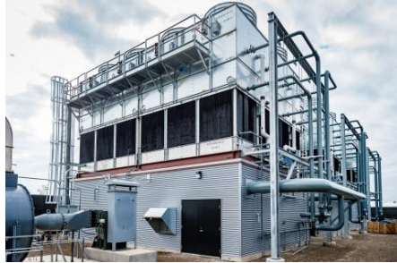
[Cooling towers – 12MW]
