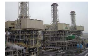
Waste Heat Recovery
