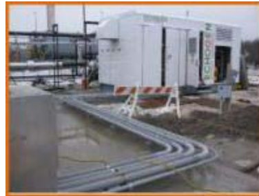
250 KW Pilot system
